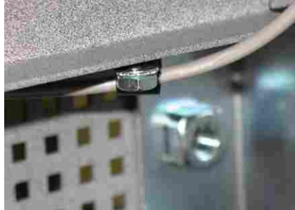
Figure 11: REMOTE Charger Data Cable Routing
