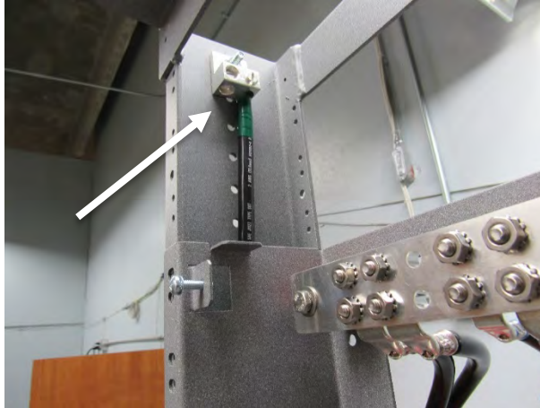
Figure 5 – Ground Lug Connection
